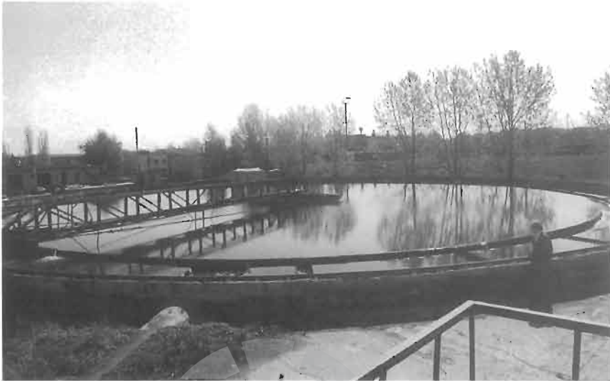
Figure 7. Clarifier used in a wastewater treatment plant.
