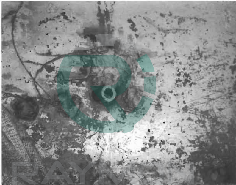
Figure 16. Shows severe pitting and corrosion on the wall of a steel underground storage tank.
