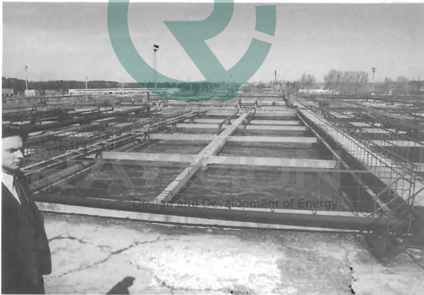
Figure 8. Rectangular settling basins in operation.
