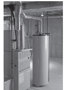
Heating systems © Comstock RF
