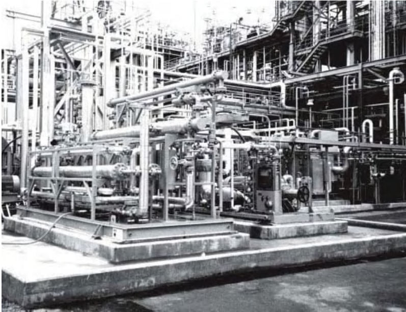
Figure 8.37 Photograph of a membrane unit used to recover nitrogen and propylene from a polypropylene plant vent gas
