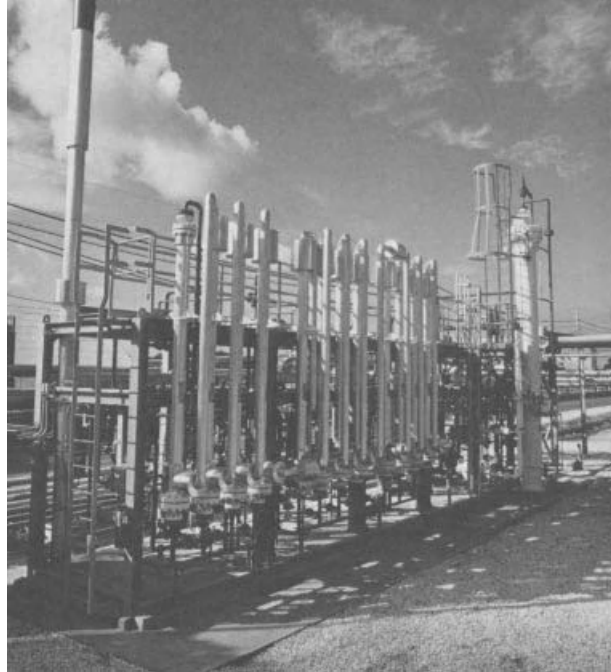
Figure 8.22 Photograph of an Air Products and Chemicals, Inc. PRISM ® membrane system installed at an ammonia plant. The modules are mounted vertically
