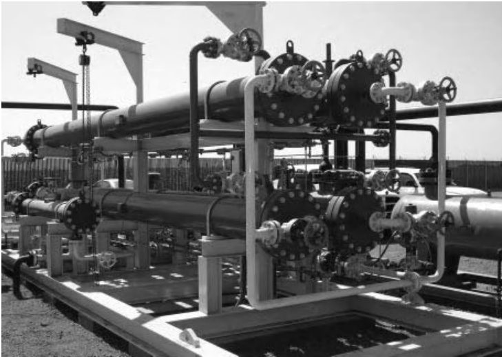
Figure 8.35 Flow diagram and a photograph of one of the two membrane skids at a 12 MMscfd membrane nitrogen removal plant installed on a high-nitrogen gas well in the Sacramento River Delta region of California
